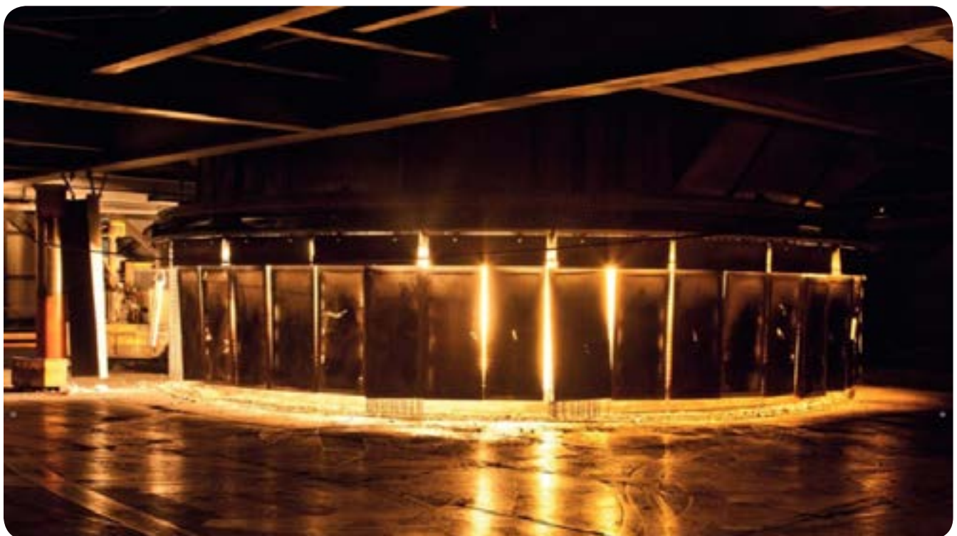
Figure B3.4 Electric submerged arc furnace producing high grade silicon used in solar cells
